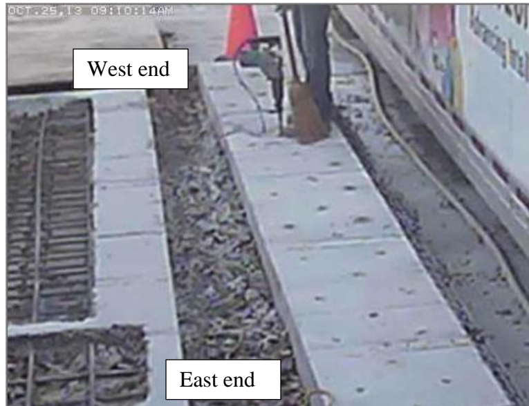
Figure 15. A photograph of drilling and cleaning holes taken by the networked camera
